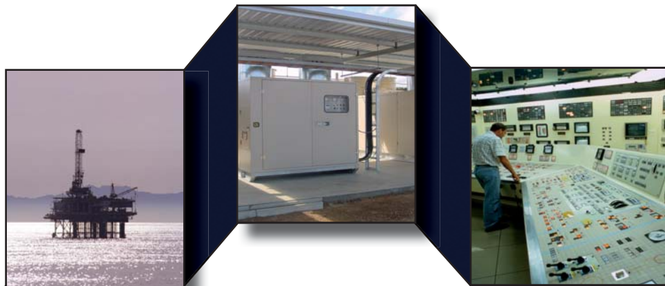
Switch & Control Rooms
